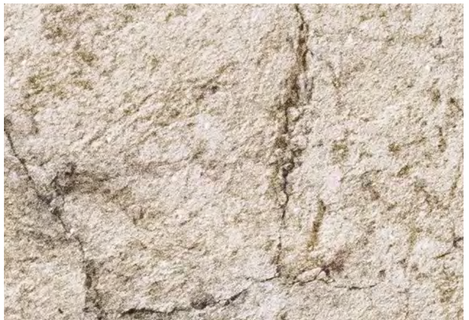
Shrinkage cracks appearing in base coats
