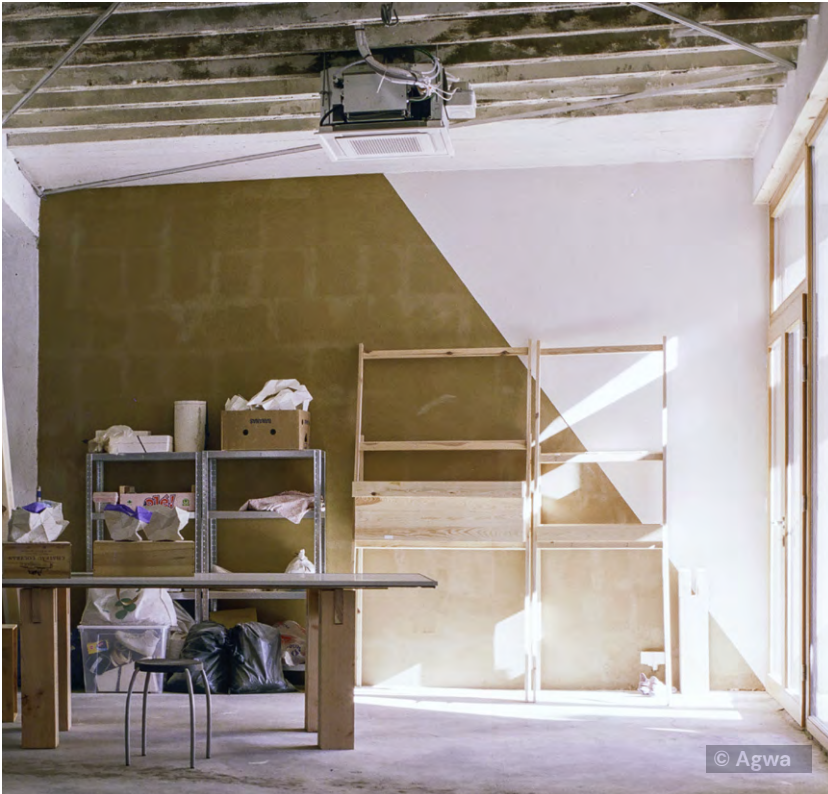
One base coat of Léem Clay Plaster Brown on top of hempcrete masonry. The ghost lines of the masonry joints shine through. To avoid this, at least two coats are needed.
