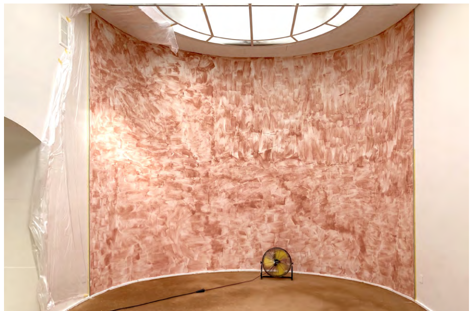
An existing gypsum substrate prepared with structured primer to allow the Léém Clay Plaster to properly anchor on the wall
