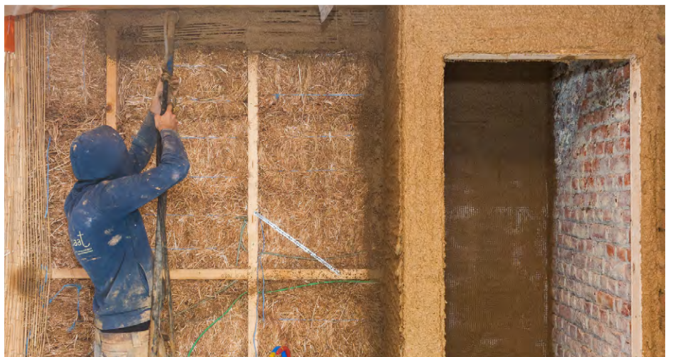
Léem Clay plaster applied with a spraying machine on reed lath, strawbale and masonry
