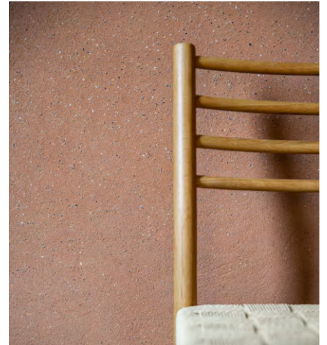
Natural sand present in the Léém Clay Plaster becomes visible as a result of excessive sponging
